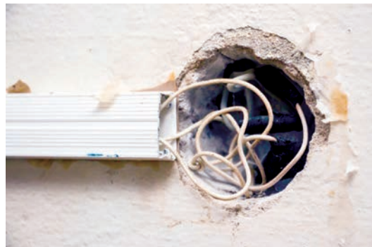
Fig. 1.28: Be careful of exposed cables
