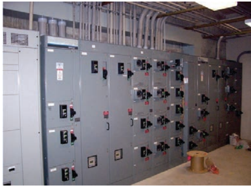
Fig.8.10 Motor control centre in control panel
