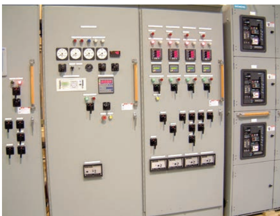
Fig. 8.8 Switch gear cabinet in control panel
