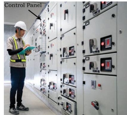
Fig.1.1(a) A wireman monitoring a control panel
