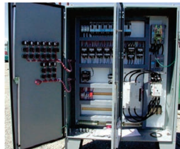
Fig. 8.26 Board inside the panel
