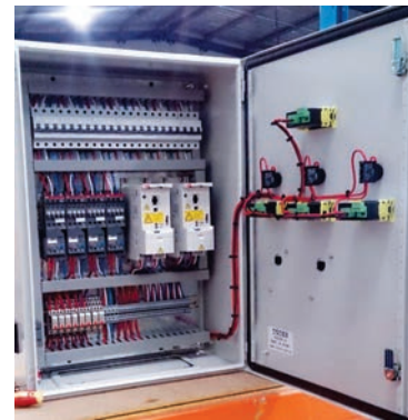
Fig. 8.17 Another way of cabling and wiring
