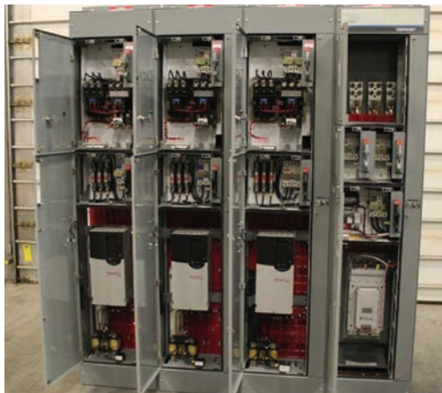
Fig. 8.11 MCC bucket centre assembly in control panel
