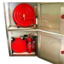
Fig 6.2.14 Fire hose cabinets
